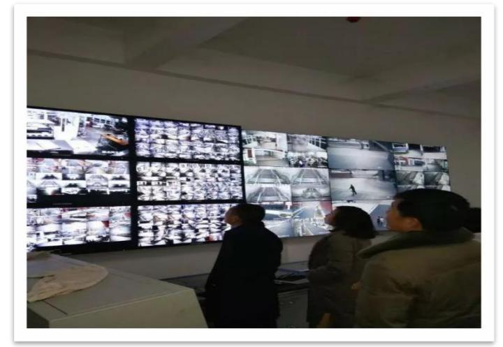
School control room
